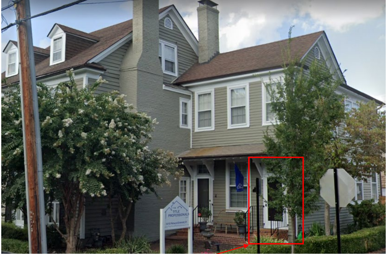
Existing aluminum storm door to be replaced.
