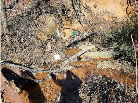
Figure 3. The inlet side of the pipes. There are two limited flow connections to the remaining system, just to the left of the white square in the foreground and near the base of the green cylinder near the center of the picture.
