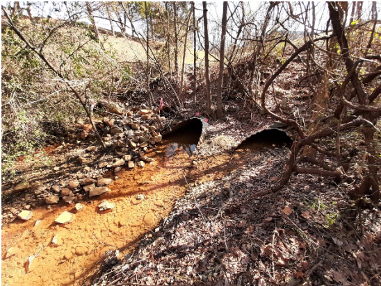
Figure 1 Outfall pipes of existing Learning Lane culvert system. Each of the 72-inch by 44-inch pipes is substantially plugged by dirt. The third culvert is barely visible to the left.
